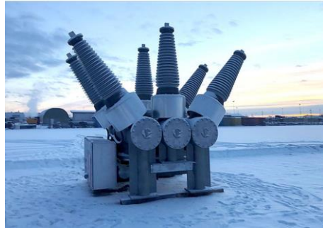
Meidensha 145 kV vacuum + technical air in Alaska
